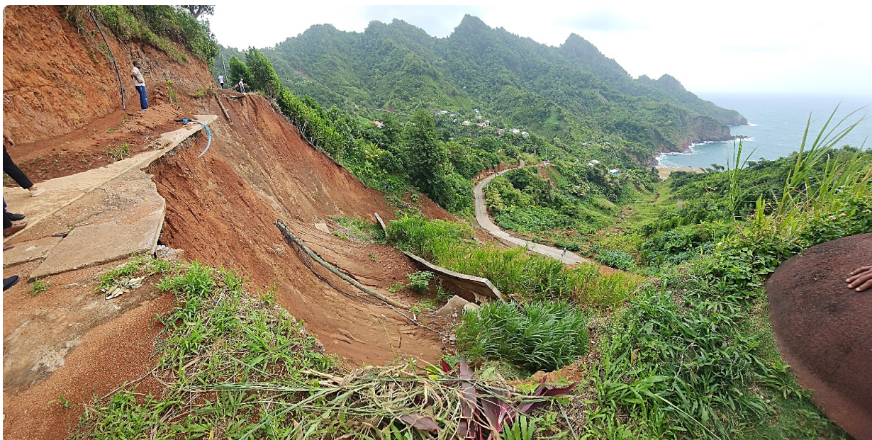
Site of the major landslide in Dominica due to intense early November 2022 rainfall, where community opinions link the slide to poor road/water drainage planning in a landscape that epitomizes ridge-to-reef (Photo: EbA Project).
